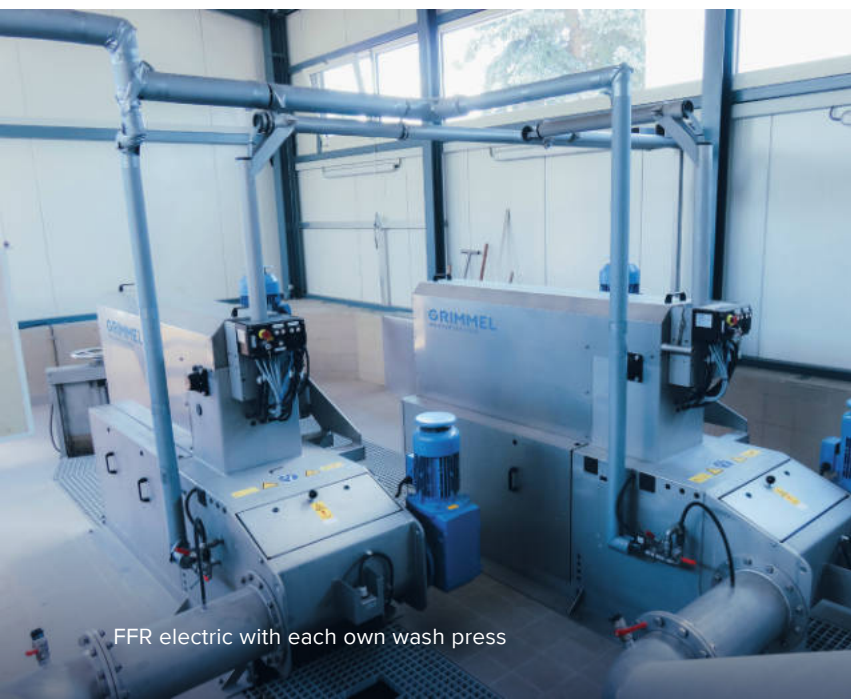
FFR hydraulic with combined wash press
